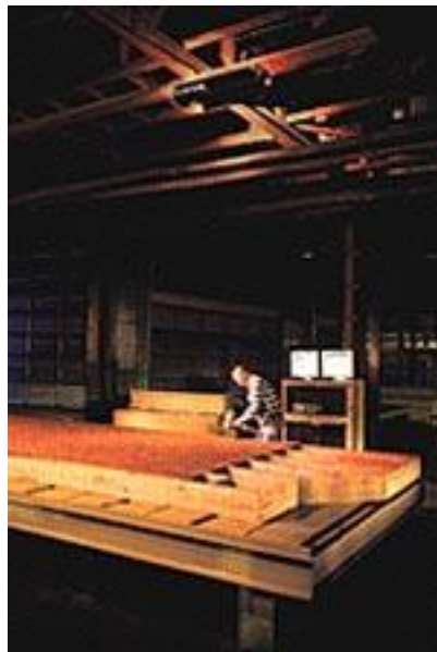
Figure 19: Projection System Used for Templating Purposes. Here a laser system is used to project the pattern onto large piecework. Later in the process, parts can be inspected using a different laser system. (Image: Virtek Vision International, Inc.)
